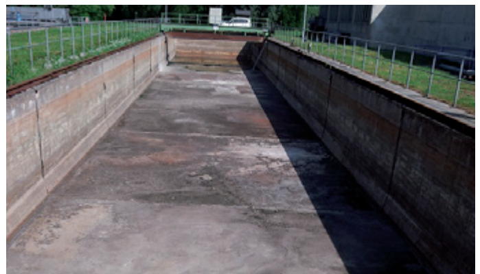
Buffer tank before refurbishment
