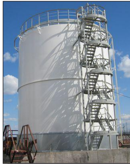
Storage tank for jet fuel
