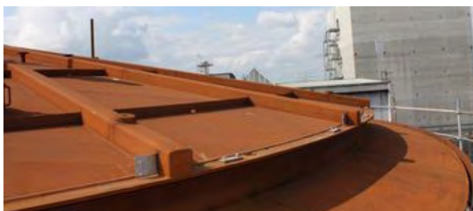
The corroded roof area of the tanks after buildup.
