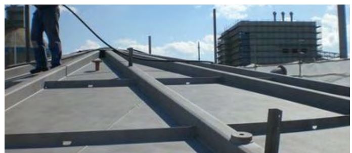
The roof surface after professional preparation by sand blasting according to ISO 8501-1.
