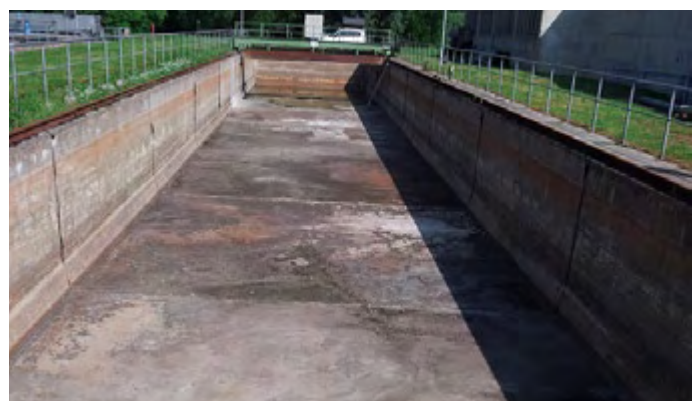
Buffer tank before refurbishment
