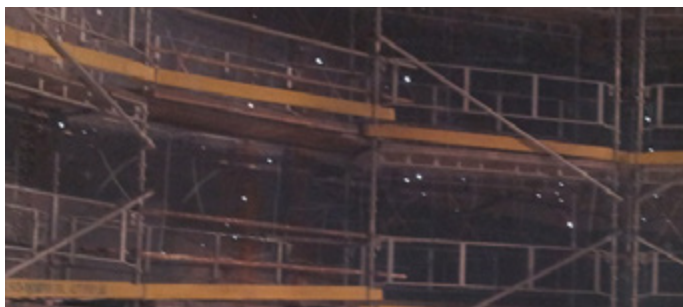
Before the restoration: Clearly visible perforation corrosion. The company ISDW sealed the holes and laminated the damaged spots with glass fiber.
