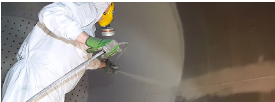
Simple application of PROGUARD CN 200 using airless sprayer. On this picture you can see that the welding seams were pre-treated with the coating within the preparatory works.
