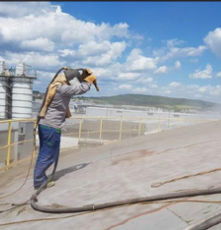
The roof area was prepared by sandblasting pursuant to purity level Sa2.5.
