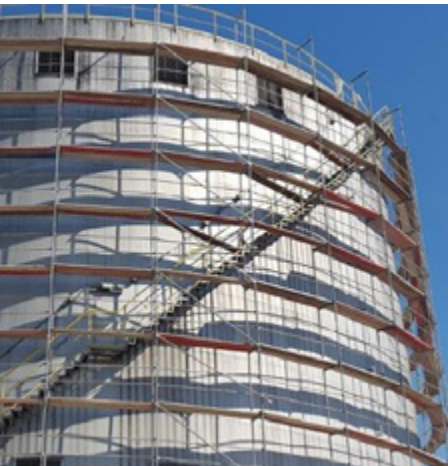
A thin layer of both coating and top coat was simply applied by airless spraying.
