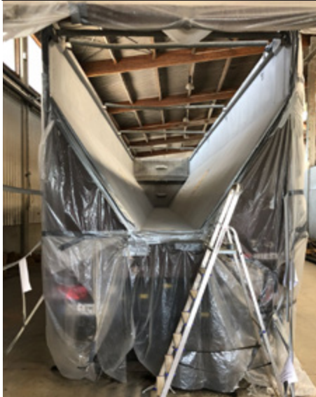
Preparation: The aluminum substrate is blasted according to purity level of minimum SA 2,5 with a roughness profile of 100-120 µm.
